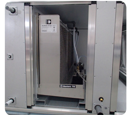
Example of an FA6 installation in a section of an airhandling unit.
